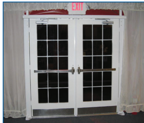
Interior View With Panic Hardware
